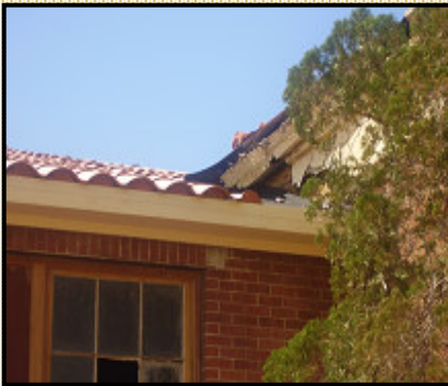
Severe masonry damage on the roof.
