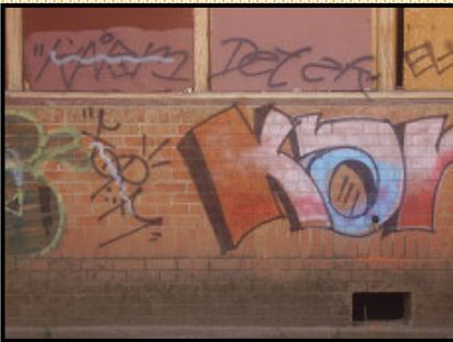
Complicating the tuck-pointing was graffiti on the north and east walls.
