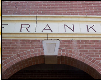
Archway keystone broken along stair-step crack from top of building.
